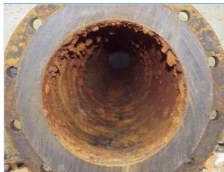
Figure 1: Mass loss due to pipe corrosion
